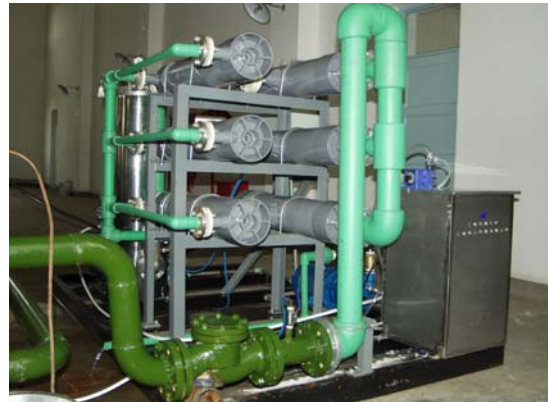
A Liqui-Cel® Contactor System built for Boiler Degassing by Shen Lan
